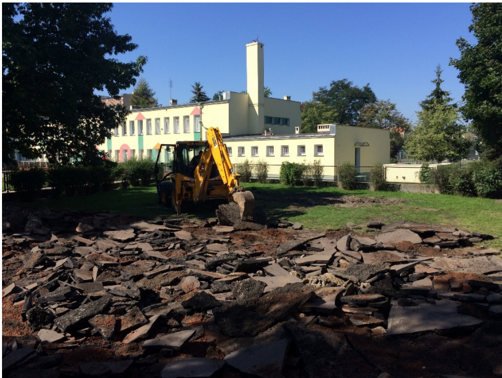
Pic. no. 8 The surface in the garden for 60 years was covered by asphalt which was demolished during our modernization work (May/June, 2017).
