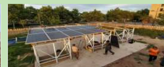
The structure has solar panels installed by the associations too
